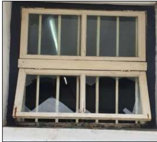
Figure 12. Broken window at The Sweetest Thing restaurant.
