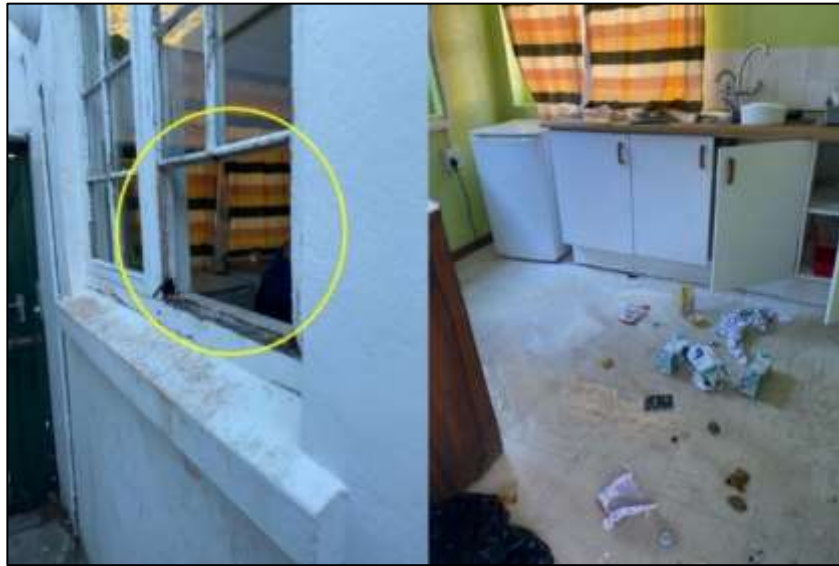
Figure 6. A baboon broke the window to gain access to the interior of this kitchen at Chrysalis Academy.
