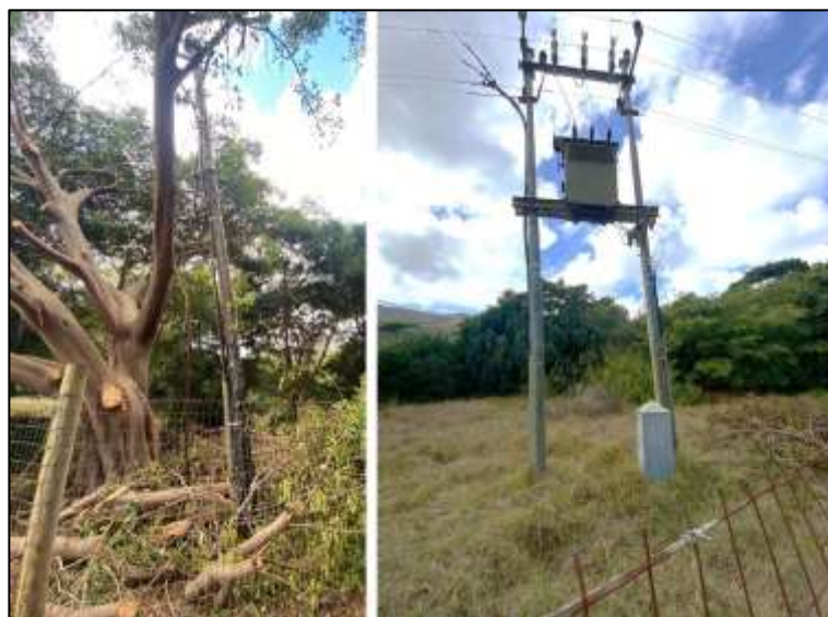
Figure 15. Greasing of electrical poles and removal of vegetation at Berg Farm to reduce the risk of baboon electrocutions.
